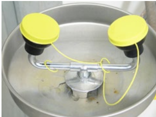
Figure 2. Eyewash with protective covers.
