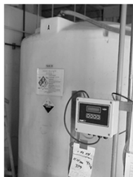
Ferric Sulfate Tank
