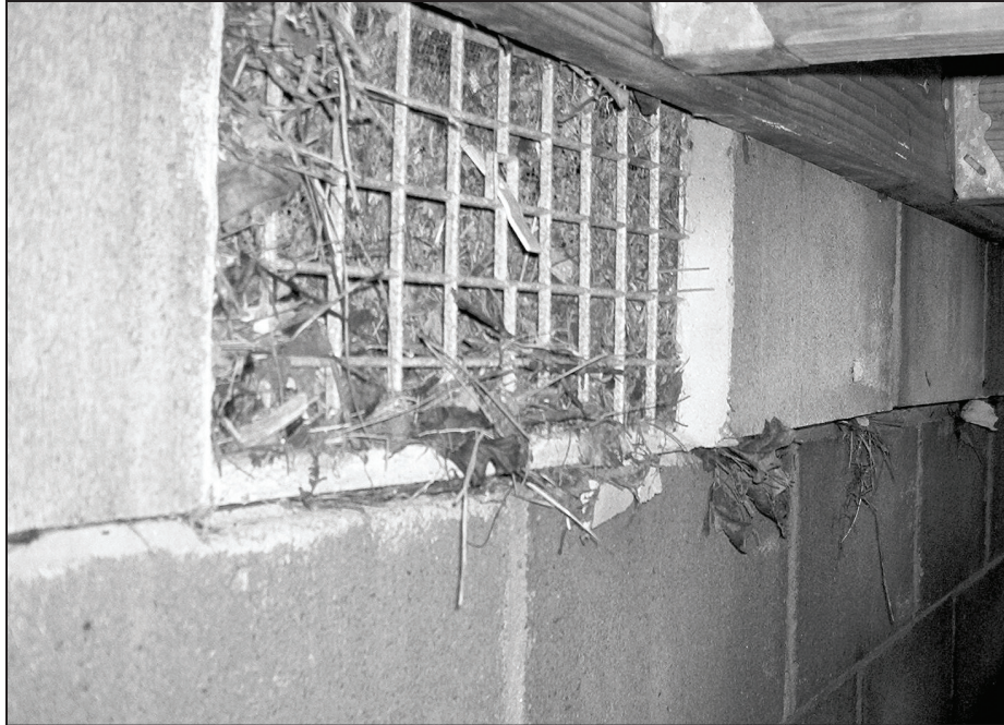
Figure 15. Typical air vent clogged by flood debris
