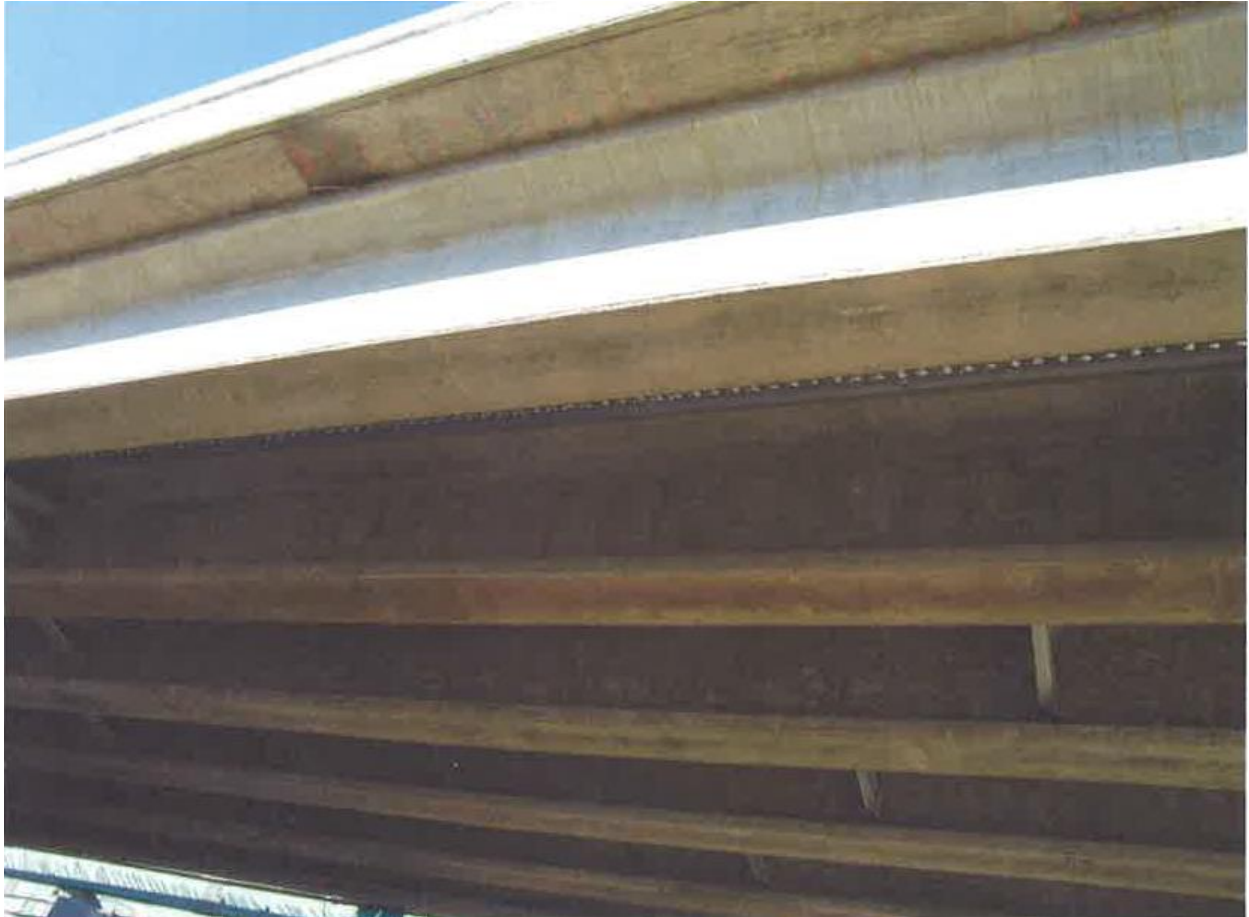
Photo 2 of 2 - Victim and co-worker were removing bolts from the top of the easternmost concrete bulb tee beam. The bolts were used to support a catwalk along the easternmost edge of the Hwy 22 Bridge
