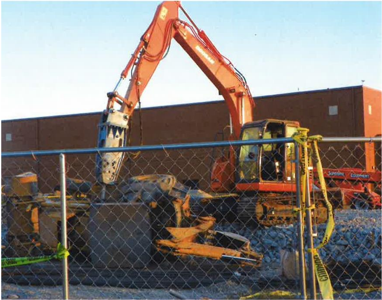
Photo 1 of 1: Track-hoe was used to move overturned back-hoe
