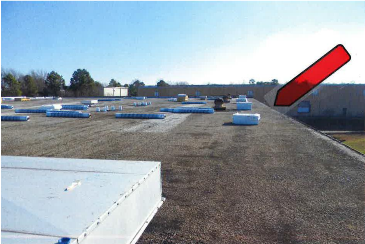
Photo 1 of 1: Red arrow indicates where the employee fell off the roof
