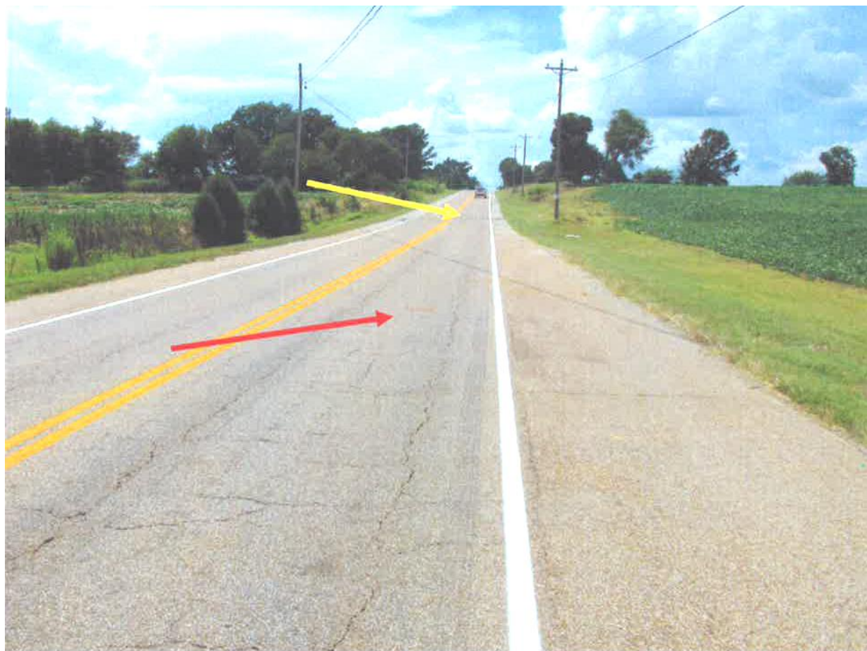
Photo 1 of 1 – The red arrow indicates the location of impact, and the yellow arrow indicates the location of the road maintenance.
