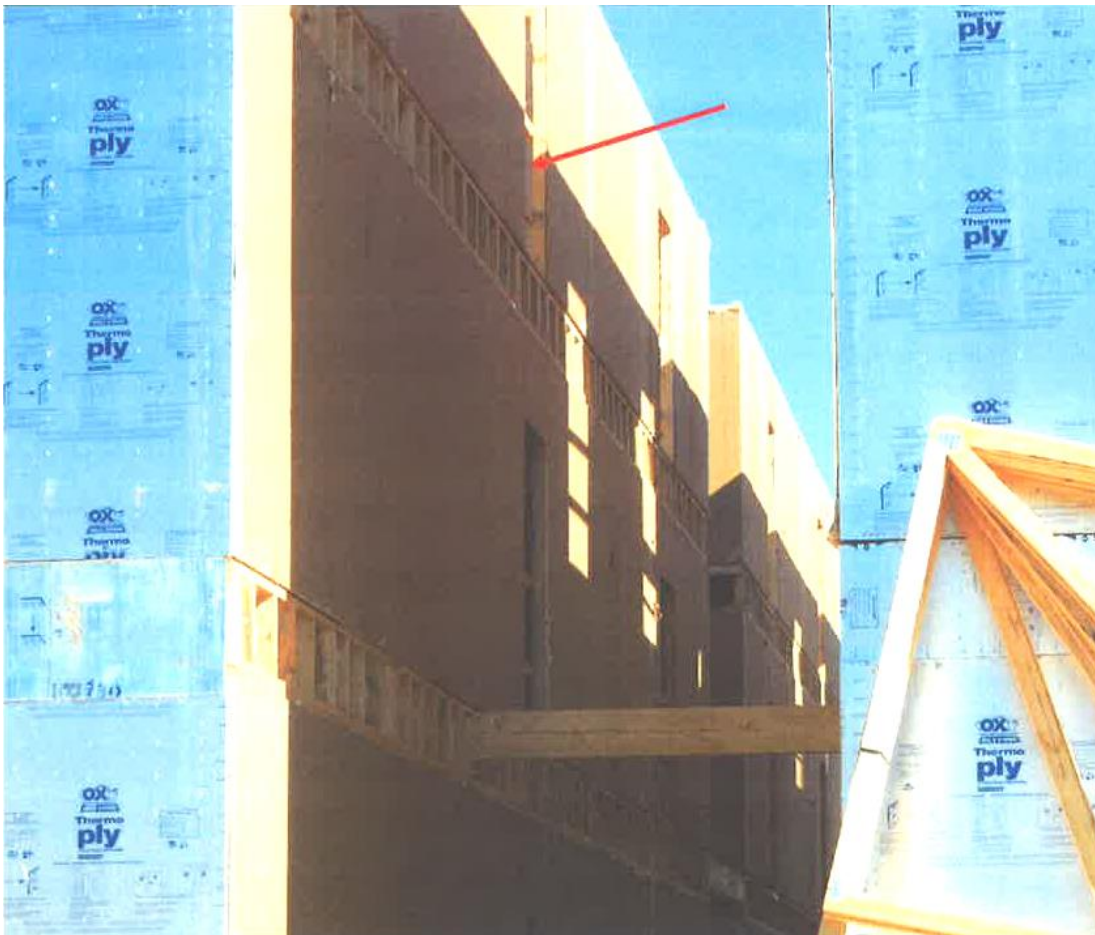
Photo 1 of 1 – A framing employee fell approximately 21 feet from a third floor door opening indicated by the red arrow.
