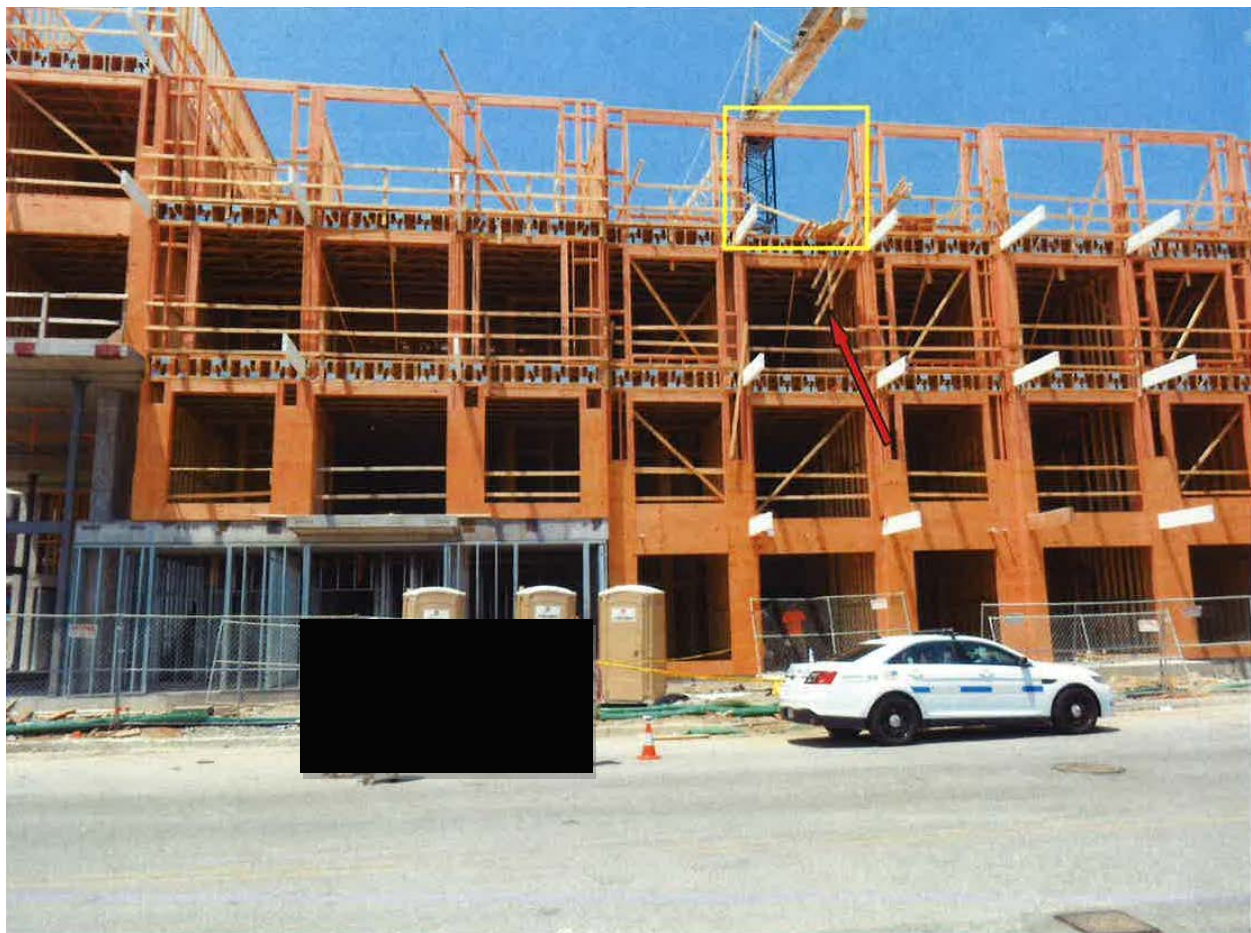
Photo 1 of 1 – The yellow box indicates the section where the railing was cut with a circular saw by the victim. The red arrow indicates the pieces of railing that collapsed.
