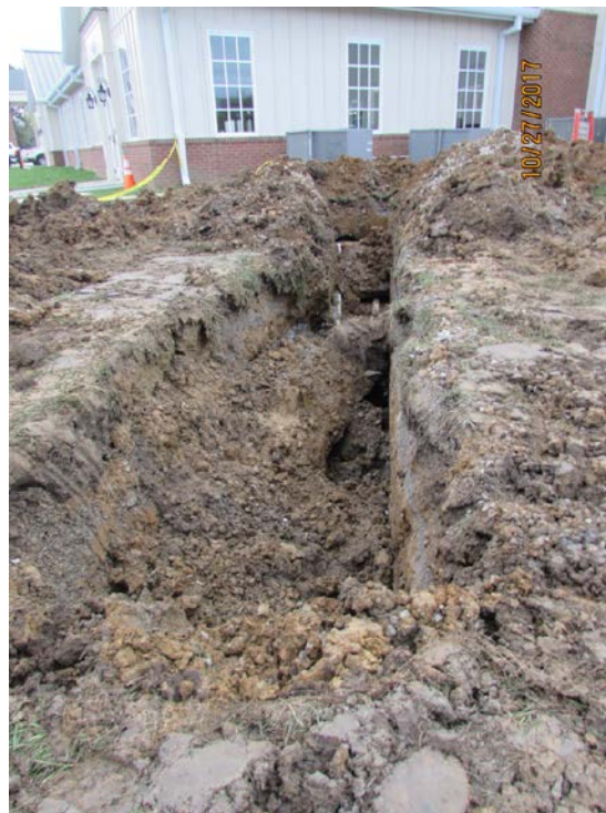
Photo 1 of 1 – Photo shows the collapsed trench.
