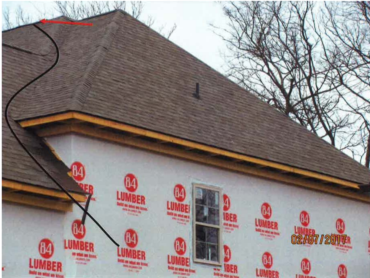
Photo 1 of 2 – The red arrow indicates the location of the roofer, and the black line indicates the possible path of the Grip Rite Eave & Valley Protector waterproofing rolling off the roof striking the victim.
