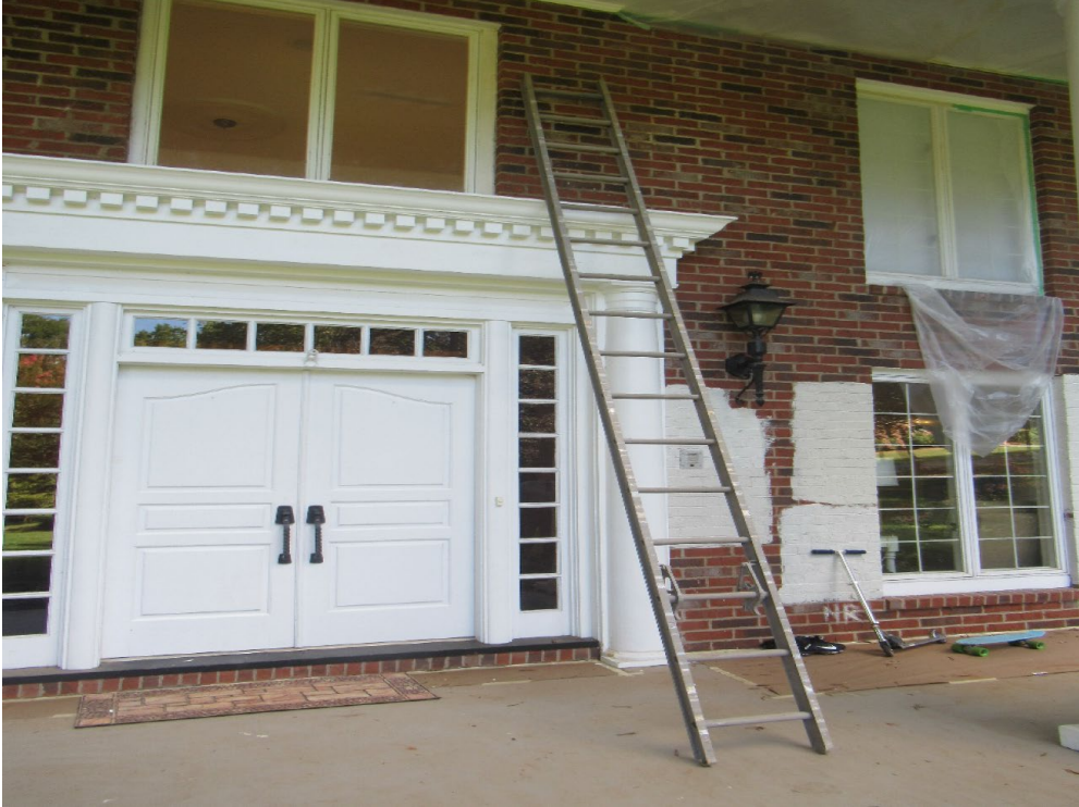
27 Fall from ladder--Insp#1489679 Early Bird Paint & Construction
