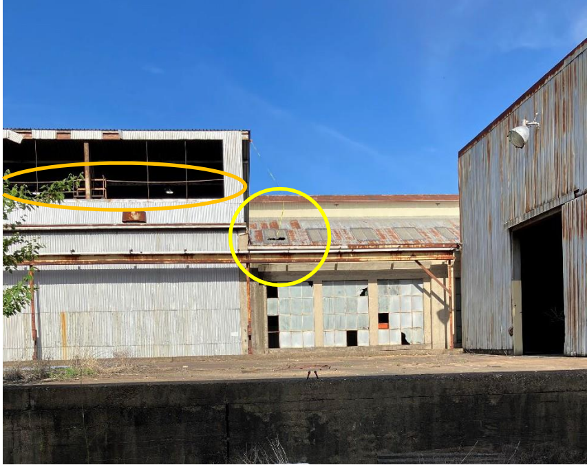
Fall through skylight—Insp # 1668035 GDL Metal Buildings, LLC
