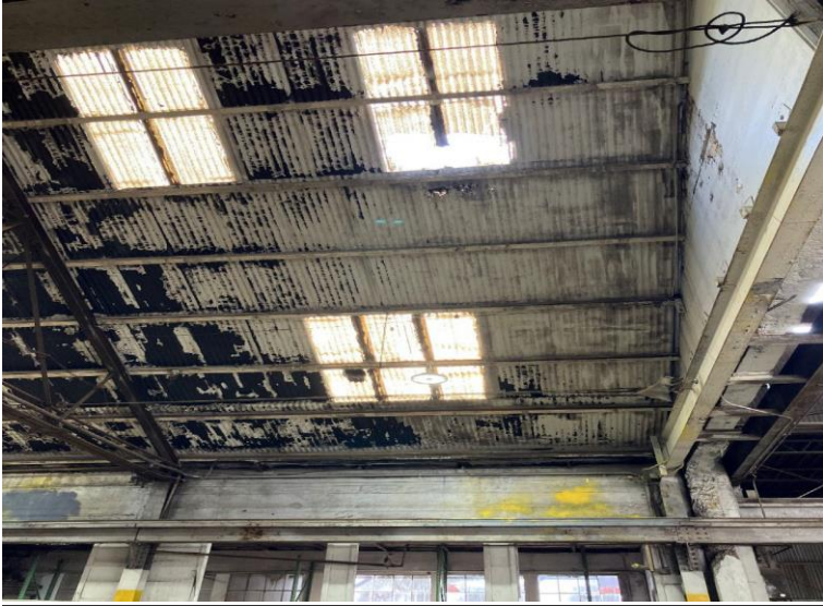
Fall though skylight—Insp # 1668035 GDL Metal Buildings, LLC
