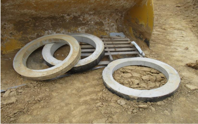
Crushed inside a concrete manhole—Insp # 1671601 Woods Construction Services, LLC
